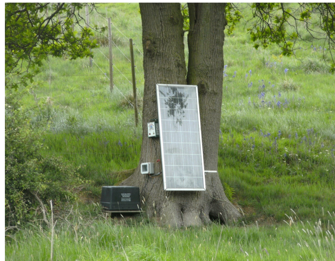
Solar powered deer fencing at
