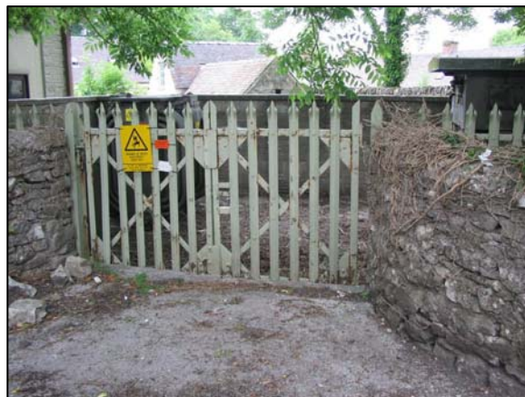
P129 Electricity sub-station by Memorial Hall
