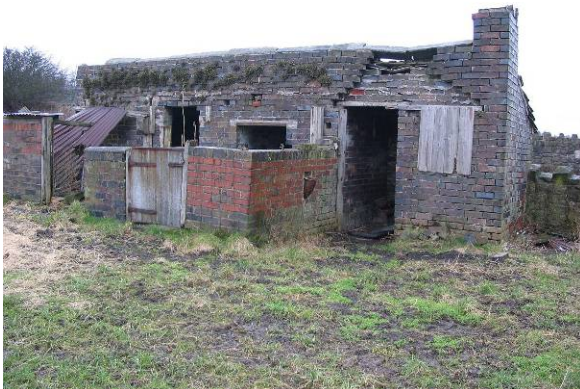
P11 Dilapidated pigsties near Town Head
