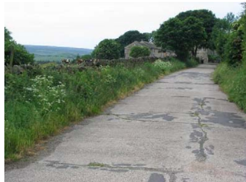
P28 Looking towards Town Head from Well Bank end of the concrete link road
