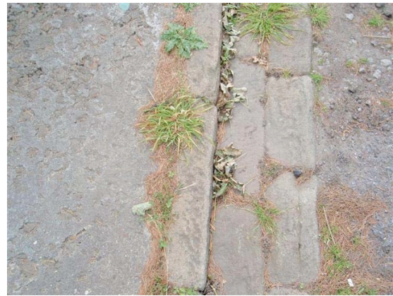
P.6.7. Stone kerbs and drainage channel to the north of the Lodge
