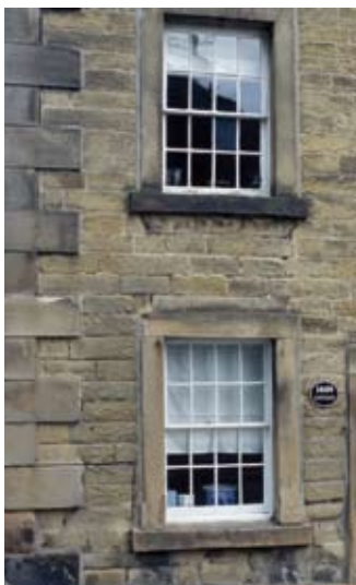
16 pane sash windows: each pane has the same vertical proportions as the window opening itself.
