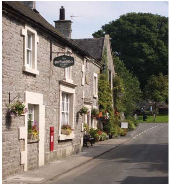
Old Post Office, Alstonefield. Altering the door into a window is preferable to creating a new opening. Irreversibly changing the door opening should be avoided
