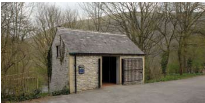
Composting toilets, White Lodge
