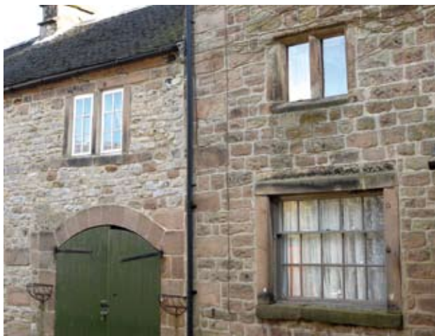
Clockwise from top right, a 17 th century mullioned window, opening, 19 th century sash window, an 18 th century mullioned window, Winster
