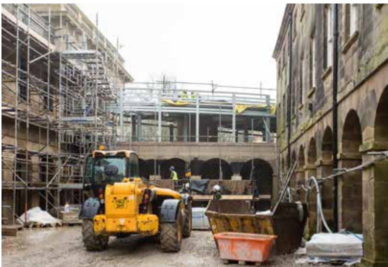
Back of the spa building (the former Natural Baths), with the new spa extension (left)
