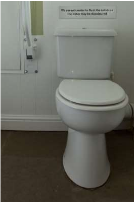
Figure 11 Rainwater harvesting for toilet flushing
