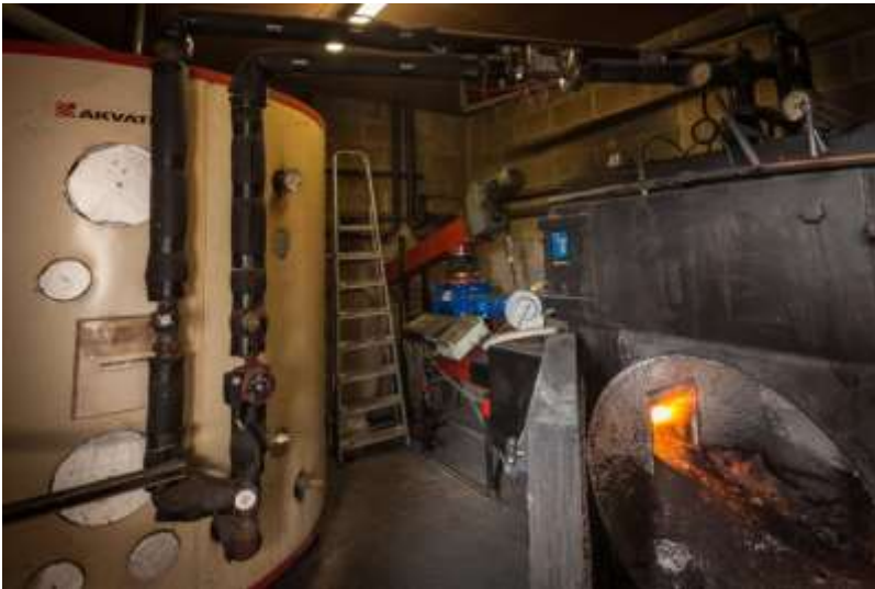
Figure 8 Wood gasification heating system and water storage cylinder
