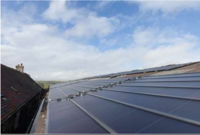
Figure 10 Photovoltaic sheeting installed on portal framed building. Location of installation minimises impact on landscape surroundings
