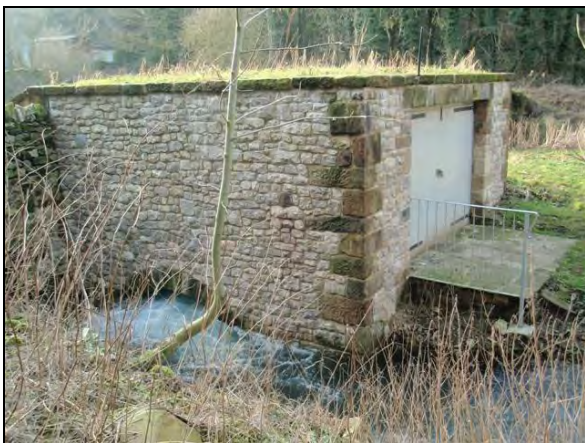
P.4.9. Water turbine house
