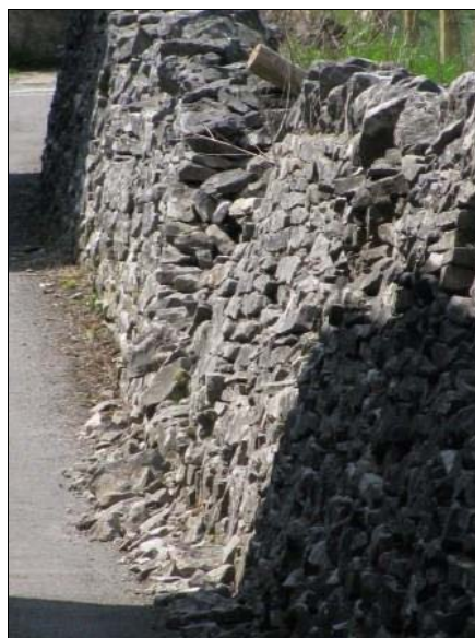
P11.1 Boundary wall on Charlotte Lane is in need of repair
