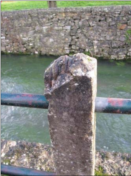
P11.4 Deteriorating concrete posts beside the stream on Brookside
