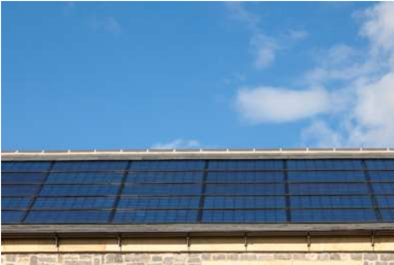
Figure 25. Flush fitted photovoltaic tiles
