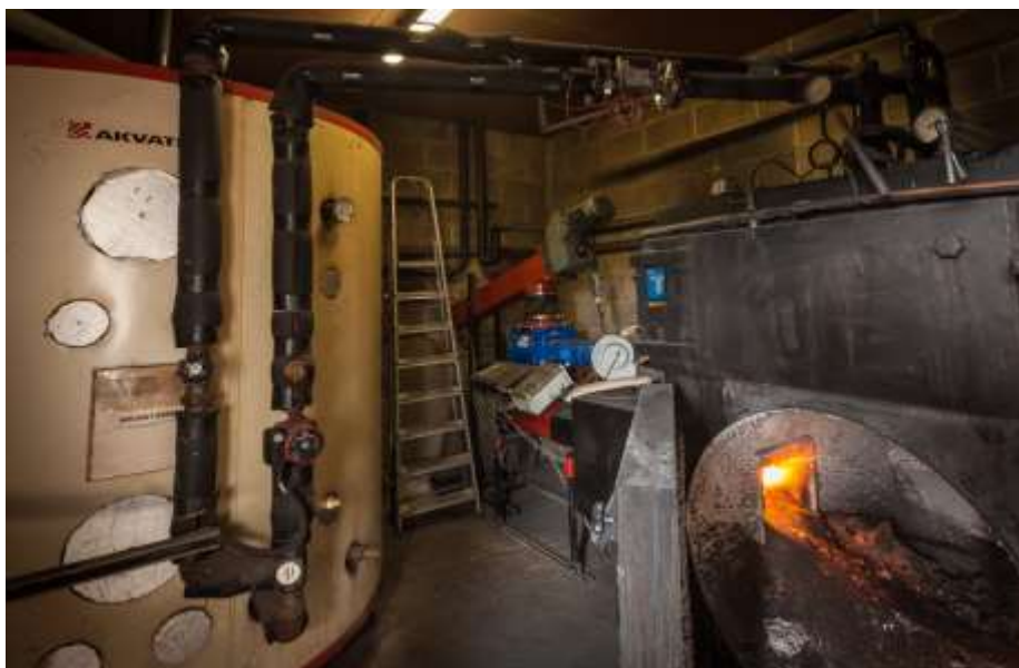
Figure 31. Mini district heating system at Beechenhill Farm
