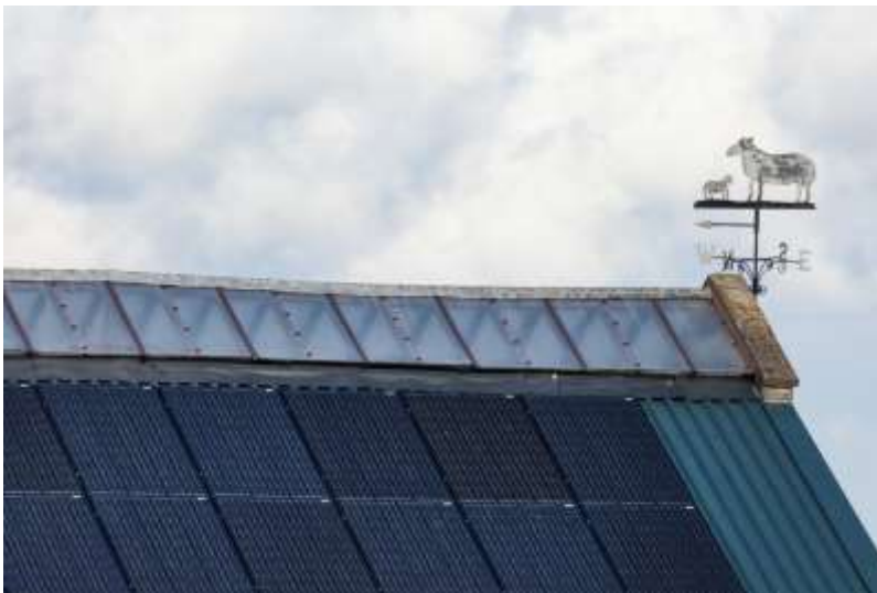
Figure 22. Photovoltaic panels on patent glazed roof
