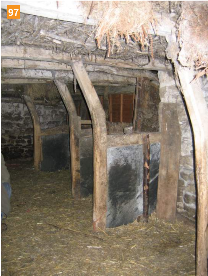
▲ 97. Slates are set into the frames of these cattle stalls, elbowed posts supporting the loft floor which here retains very rare interwoven branches of hawthorn. Photo © Jen Deadman
