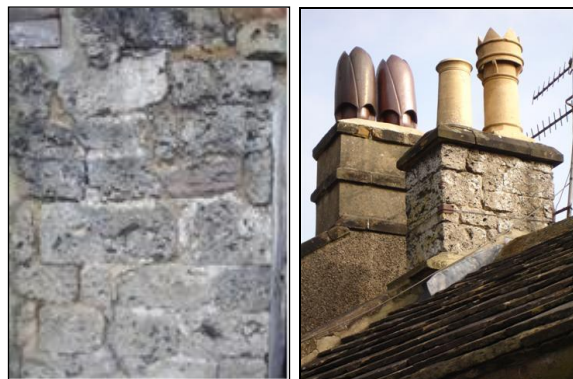
P.6.2. Left: Tufa walling to the small building south-west of the Reading Room
