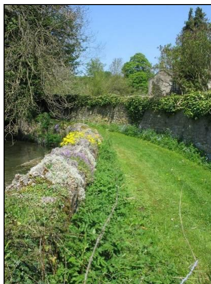
P.8.10 A combination of ivy and other plants soften the appearance of walls
