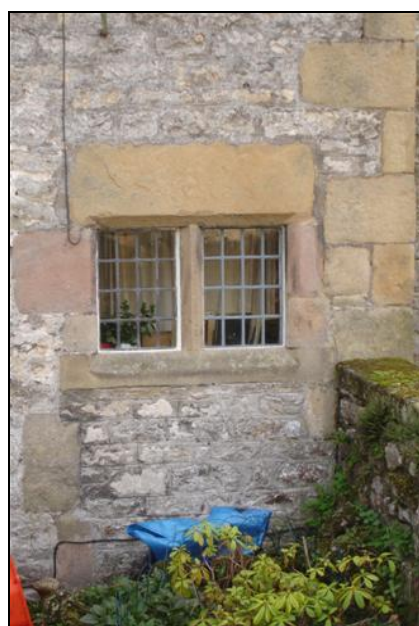
P.5.7. Blocked entrance door at Monk's Hall
