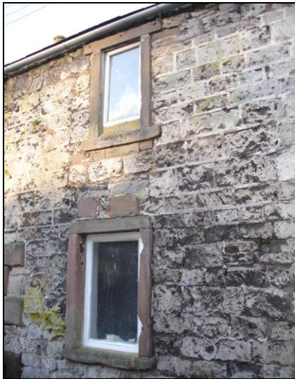
P.5.19. Window to the front of the property west of Rheinstor Cottage
