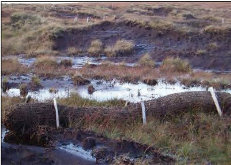
Coir rolls used to retain water and help with re-vegetating bare peat
