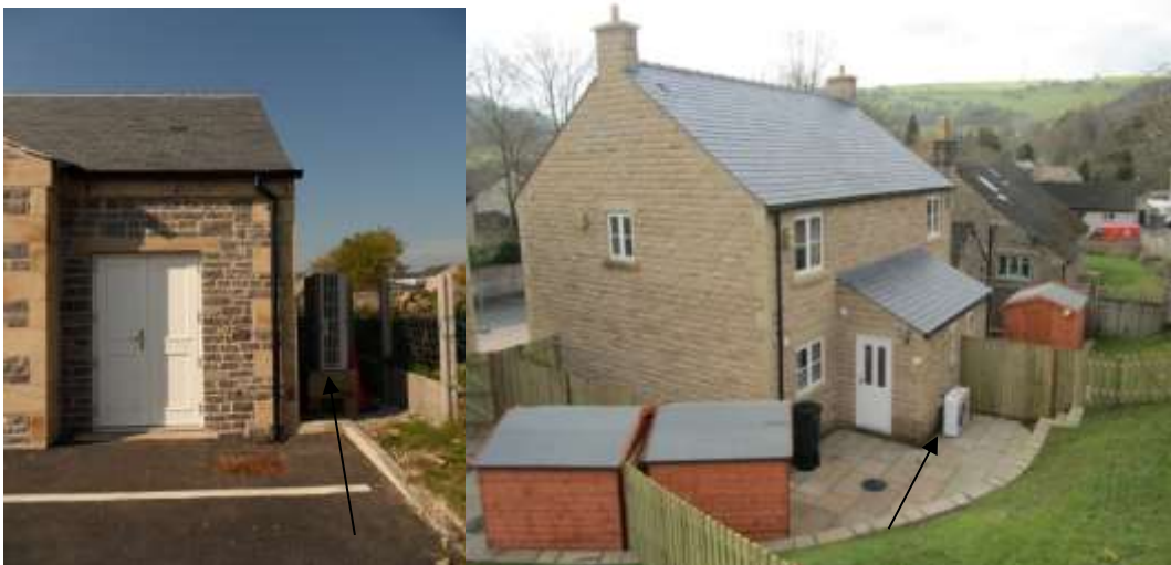
Figure 29. Air source heat pumps at Over Haddon Village Hall and on a new affordable home in Calver
