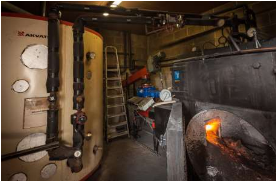
Figure 31. Mini district heating system at Beechenhill Farm
