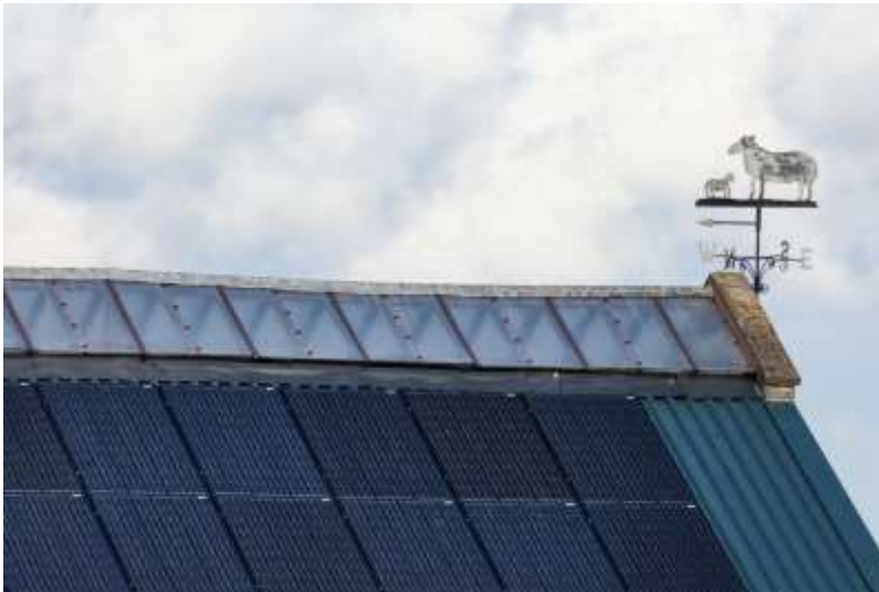
Figure 22. Photovoltaic panels on patent glazed roof
