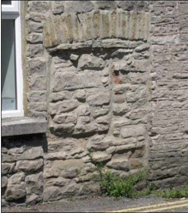
P5.6 Blocked doorway to 1 Bridge Street
