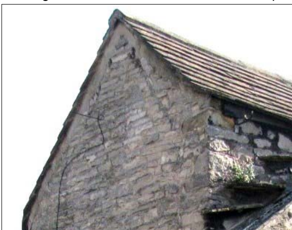
P5.3 Evidence of an earlier, more steeply pitched roof to Bradwell’s Ice-Cream Shop
