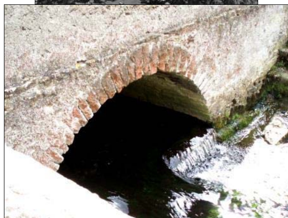
P5.52 Road bridge still with its segmental arch (top); brick arch beneath Brook House (bottom)
