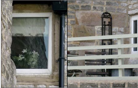
P5.15 Partially covered window at Bank Cottage (left) & door surround at Sydney Cottage (right)
