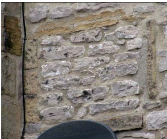
P5.19 Blocked earlier opening to Edge View, Hugh Lane
