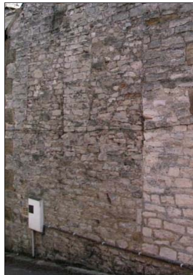
P5.14 Blocked windows to Chapel House gable
