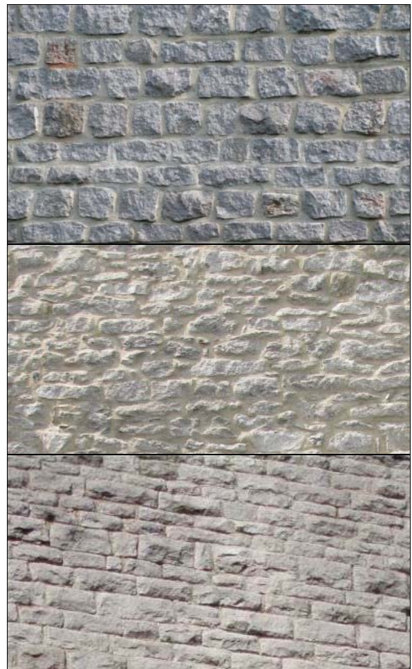
P6.2 Coursed, squared limestone (top); rubble limestone brought to courses (middle); rock-faced finish (bottom)
