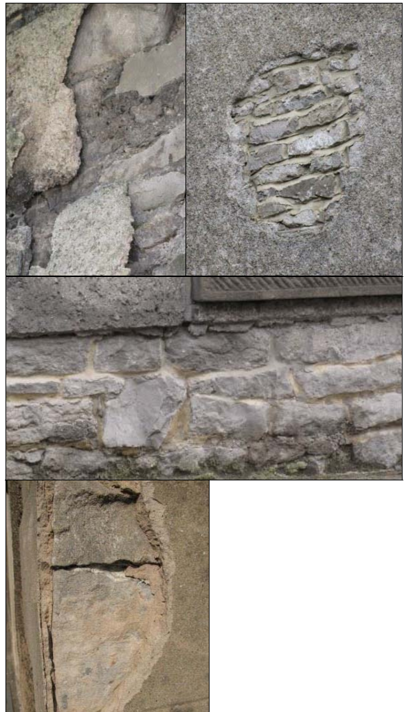
P6.6 Patches of render & cladding deteriorating to reveal stonework: Kinder Cottage, The Hills (top left); Bethlehem Chapel (top right); Bank House, Church Street (middle); Newburgh Hall (bottom)
