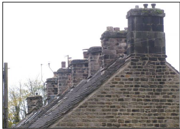
P6.3 Coursed gritstone chimney stacks with an ashlar stack on gable end
