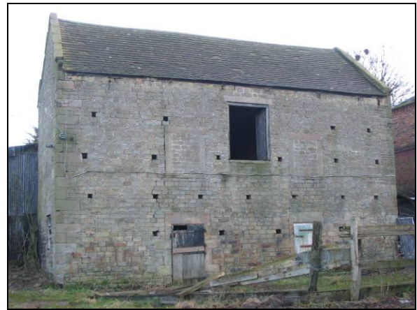
P5.13 This barn at Hall Farm, which has now been converted, originates from the early seventeenth century.
