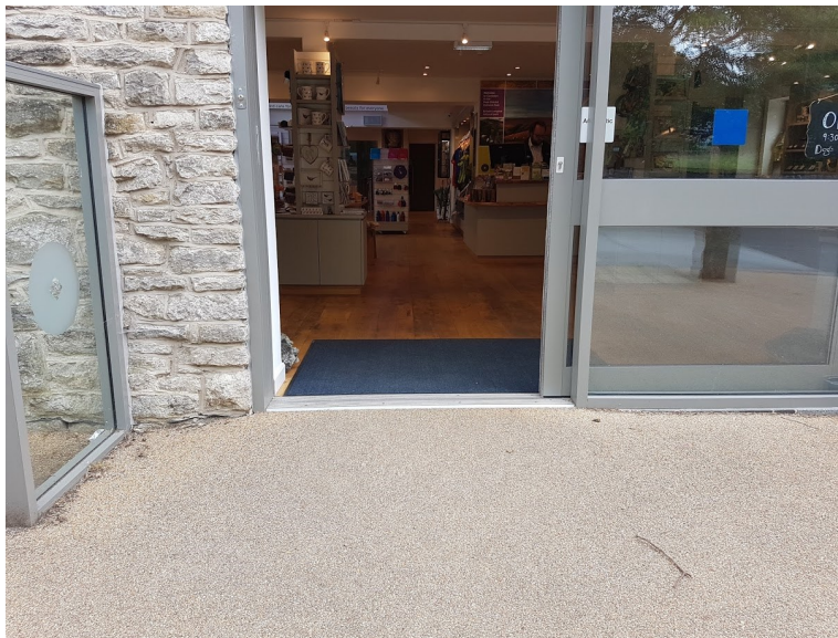
The main access in to the centre, showing a small incline on the approach to the automatic door
