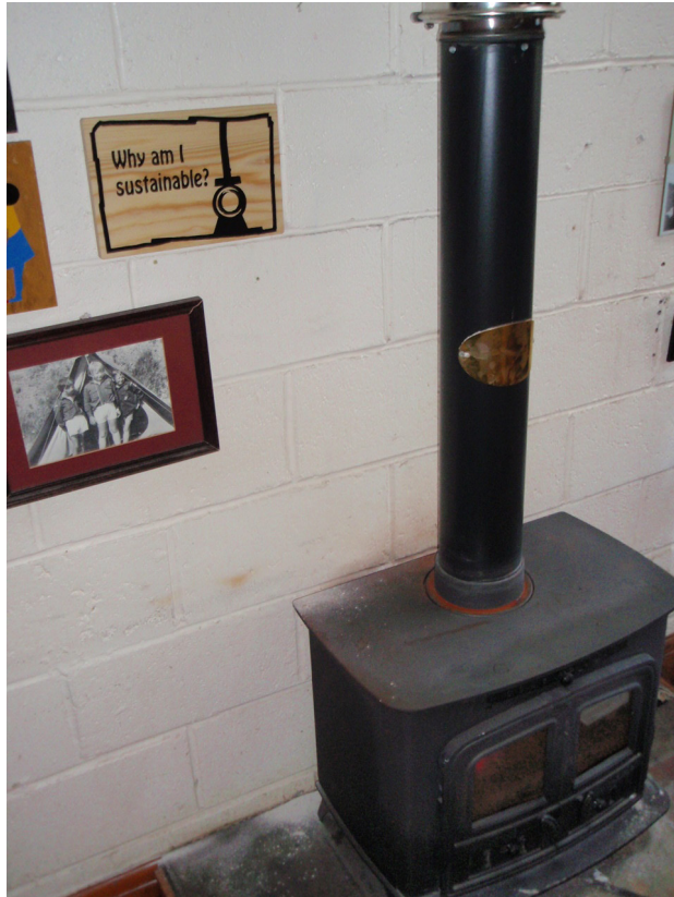
Figure 27. Wood burning stove
