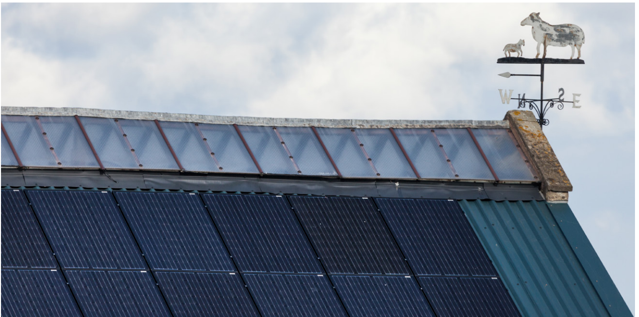
Figure 17. Photovoltaic panels on patent glazed roof
