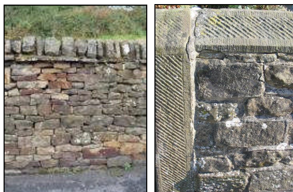
P.56 Left: Drystone wall with weathering course P.57 Right: Mortared wall with dressed copings
