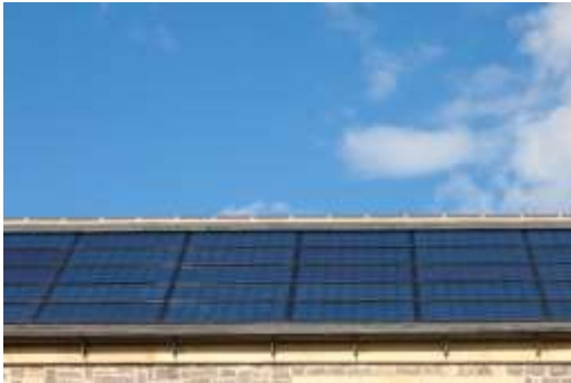
Figure 5 Solar photovoltaic panels
