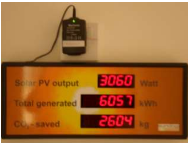
Figure 6 Monitor demonstrates benefits of system
