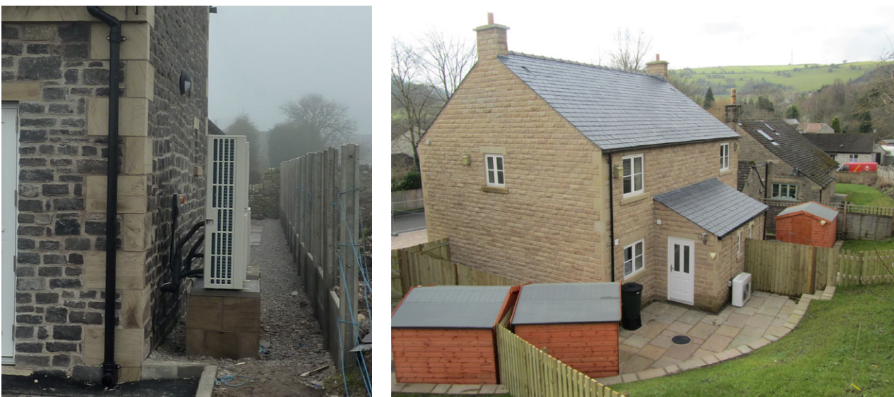
Figure 24. Air source heat pumps at Over Haddon Village Hall and on a new affordable home in Calver
