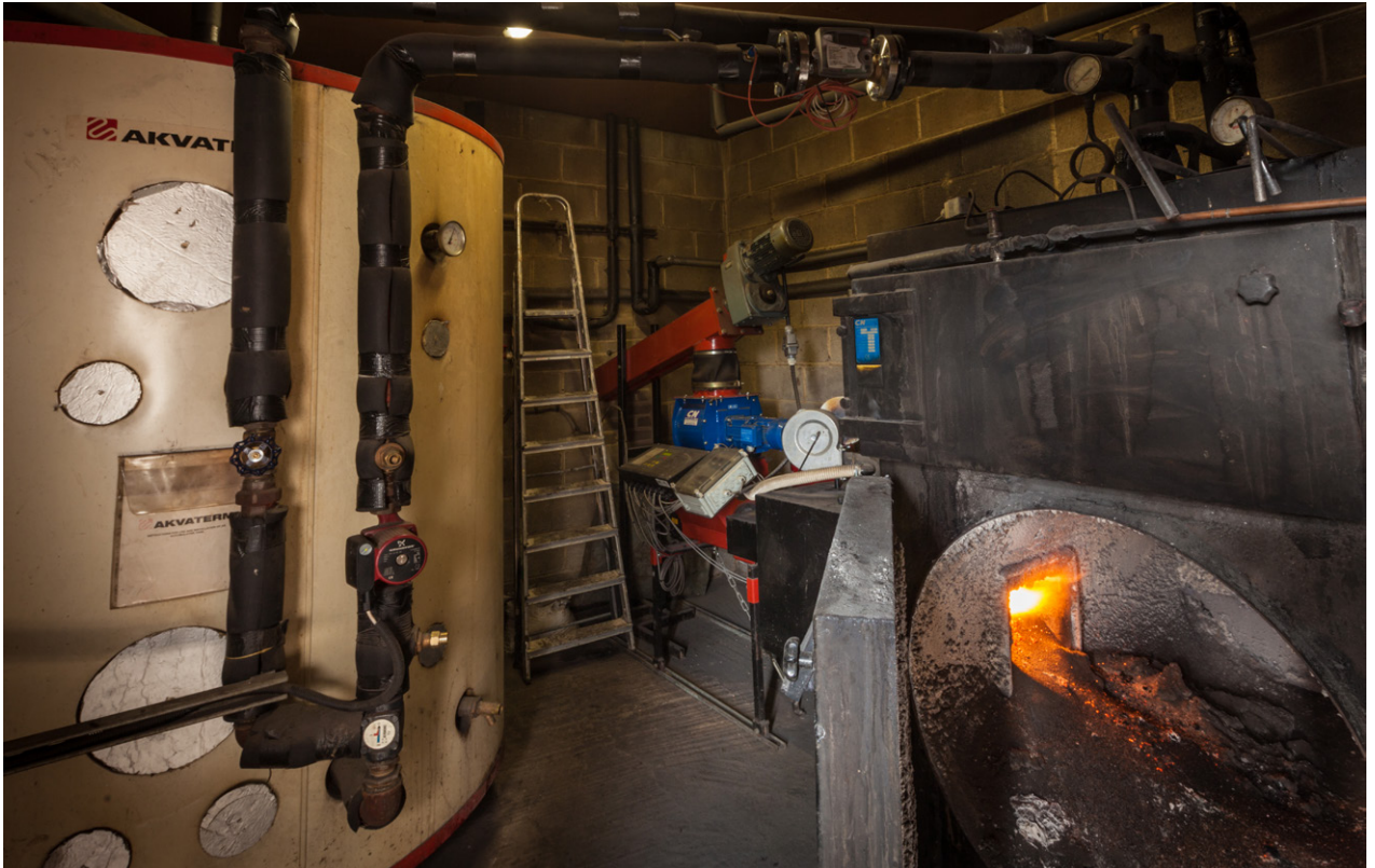
Figure 26. Mini district heating system at Beechenhill Farm
