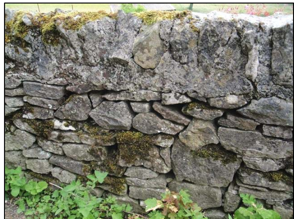
P44 Coursed, roughly coursed and uncoursed boundary walls with different coping stone details
