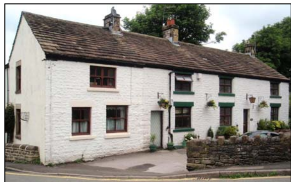
P41 Painted stonework and render to Bray Cottage
