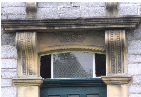
P5.7 Decorative brackets at Hawthorn House
