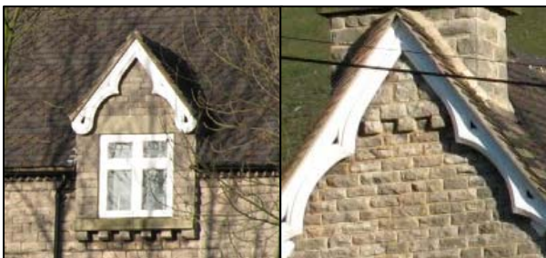
P5.17 Croft Cottage: corbelled attic dormers and stone dentil course at eaves level
