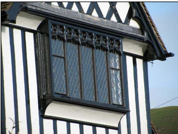
P5.14 Timber framing and oriel window, with mullions and tracery, to School House
