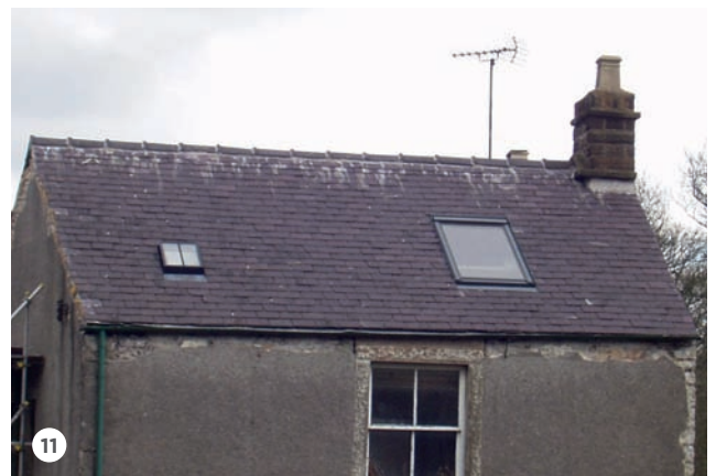
11: Size matters. The small conservation rooflight on the left looks much more appropriate on this traditional building than the oversized, modern rooflight on the right.
