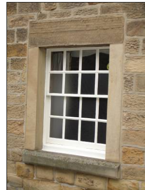
P5.27 Typical nineteenth century window surrounds with projecting sills, the window top left has a full surround with picked tooled finish. The bottom window has a double lintel
