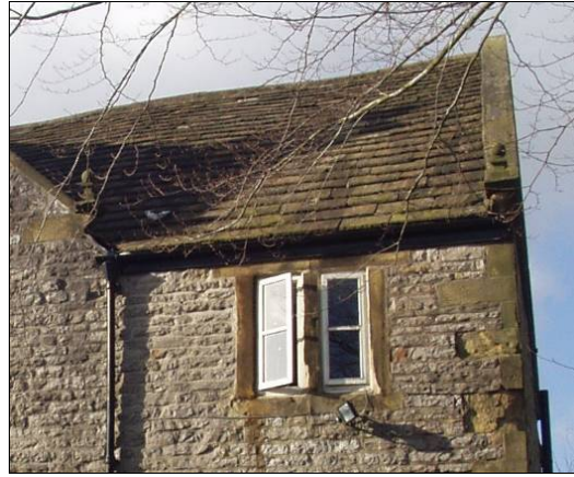
P5.17 Seventeenth century details at Bath House (note that the window surround is later, see P5.21 below)
