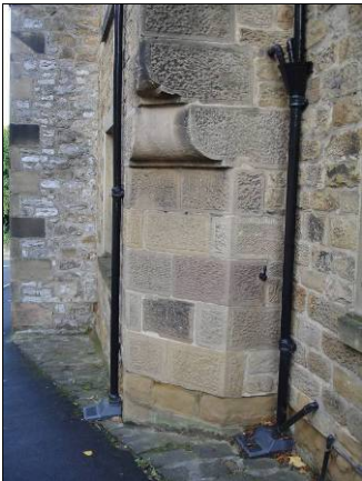
P5.29 Shaped corner details above left Matlock Street, above right, Buxton Road and below, South Church Street
