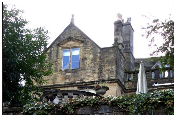
P5.13 Gable with a ball finial and window with a pediment over, Bagshaw Hall (See also P8.8)
