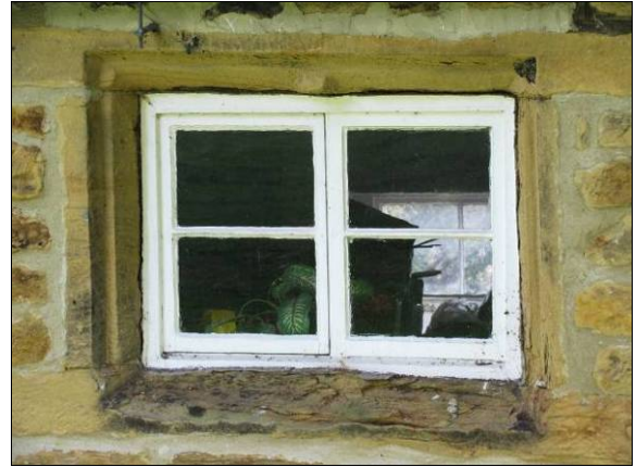
P5.9 A window surround, the mullion has been removed
