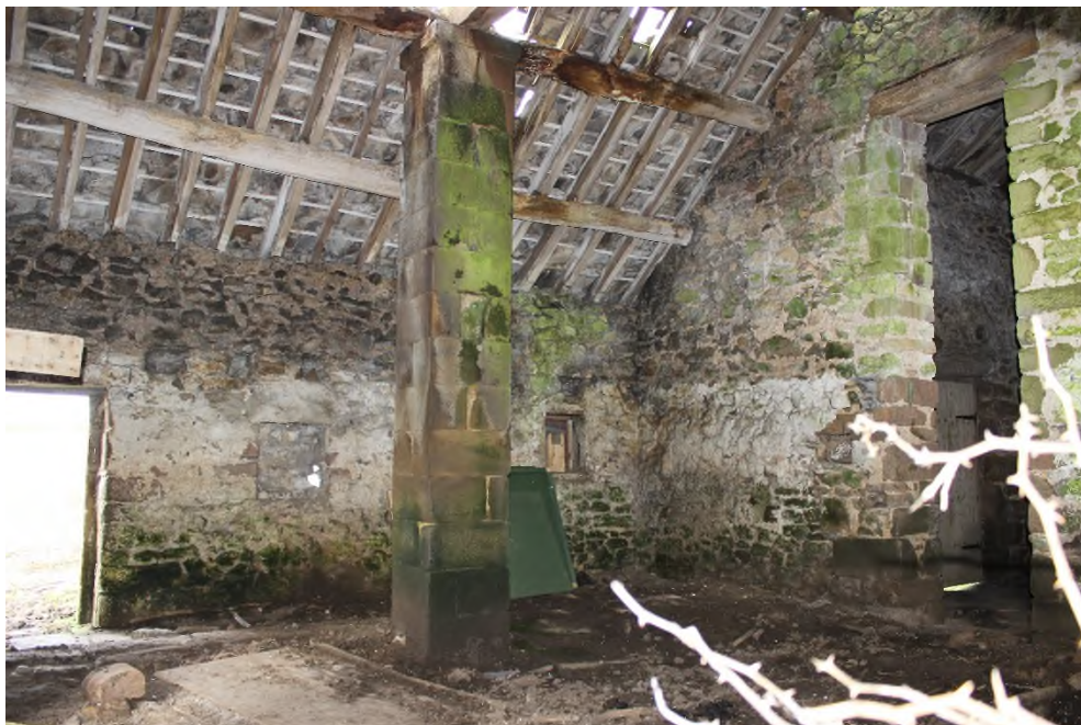
Figure 3.21 The interior of the left hand part of the field barn shown on 3.20 showing the aisled character of this part of the building.
