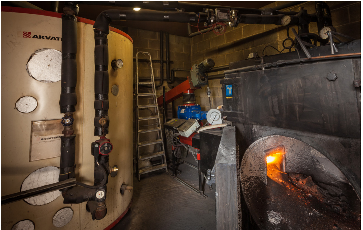
Figure 26. Mini district heating system at Beechenhill Farm
