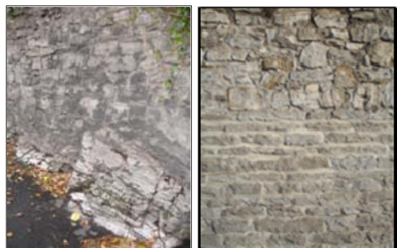
P6.13 Above Left: Limestone wall constructed on bed rock, South Church Street P6.14 Above Right: Limestone Wall, coursed to the lower part and random rubble to the upper
