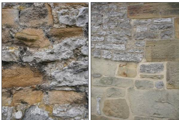
P6.15 Above Left: Limestone and gritstone wall P6.16 Above Right: Wall constructed of gritstone and limestone with gritstone quoins
