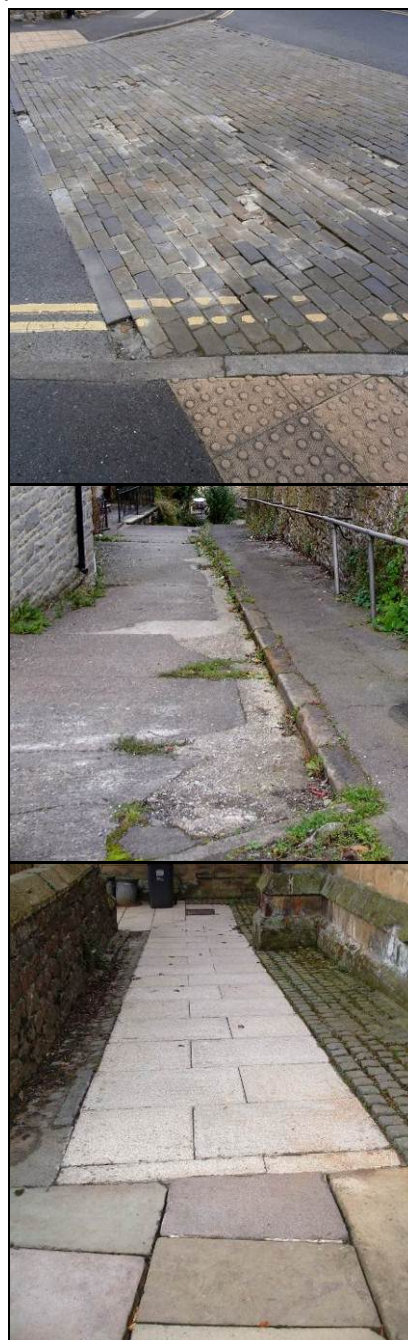
P11.7 Paving in poor condition and a mixture of paving types
