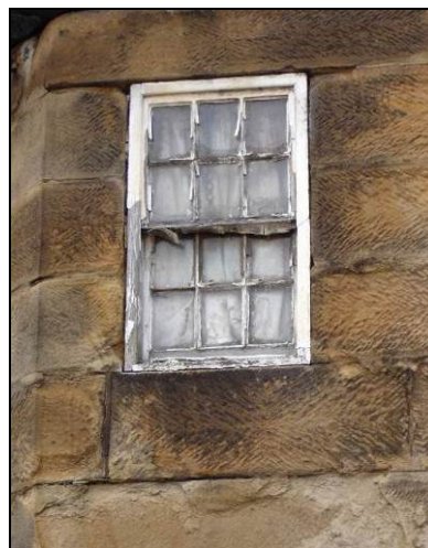
P11.1 A few buildings are in poor condition
