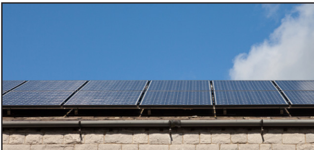
Figure 3.5 Solar photovoltaic panels
