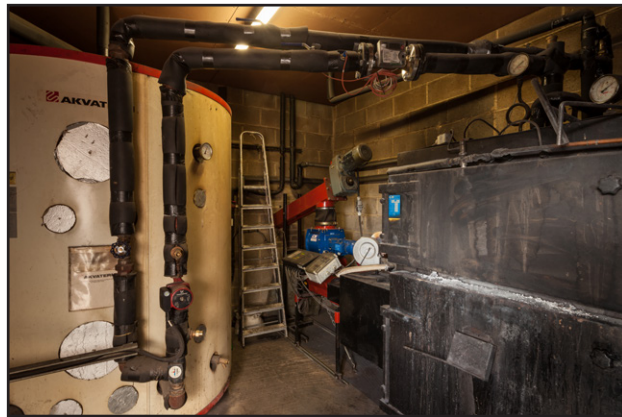
Figure 2.8 Wood gasification heating system and water storage cylinder
