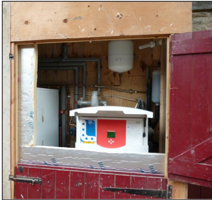
Figure 1.4 Part of the apparatus for the GSHP, also showing the levels of insulation used to prevent heat loss.
