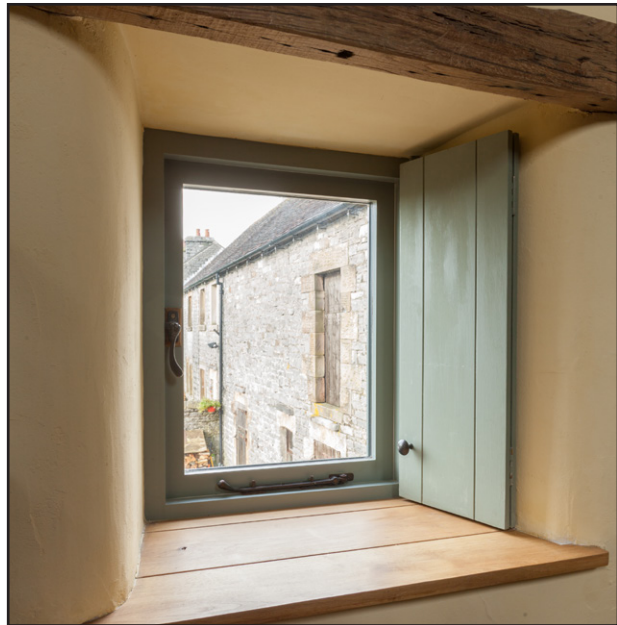
Figure 2.3 Insulated lime plaster walls conserve the internal appearance of the historic building whilst conserving energy. Home made internal shutters also conserve energy.
