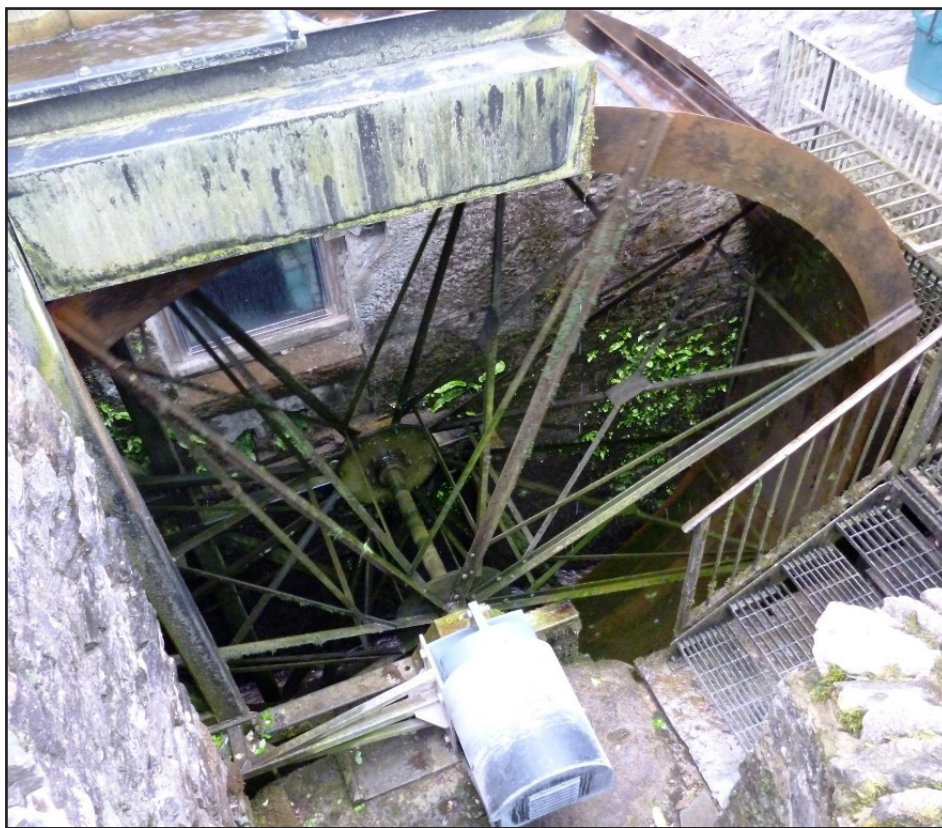
Figure 4.2 The new wheel, with its compact generator below.
