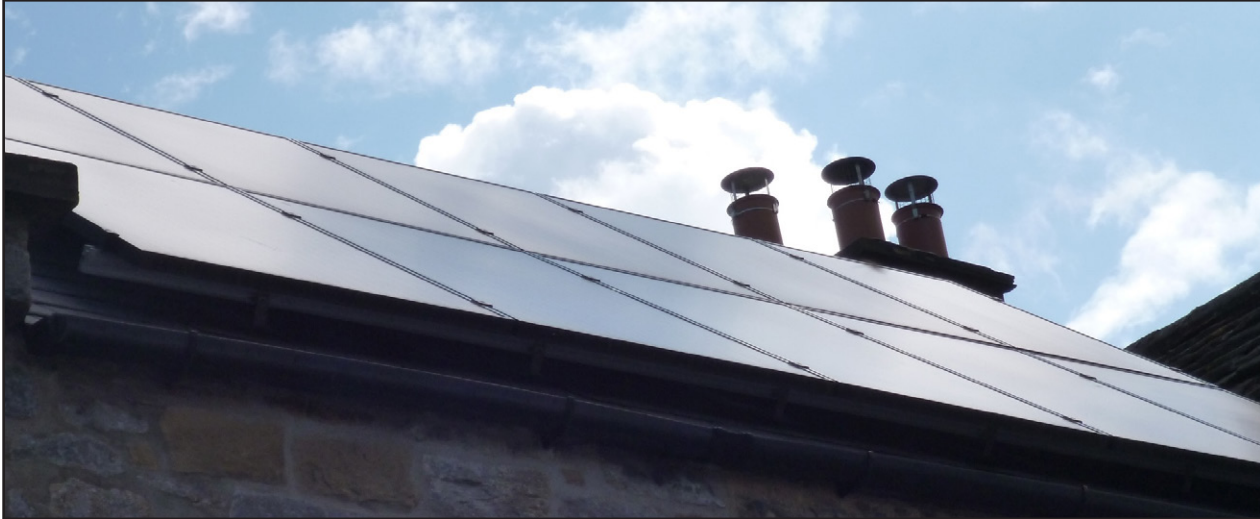
Figure 4.3 Solar panels on the roof of the building.
