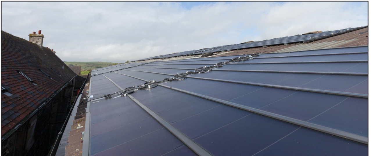
Figure 2.10 Photovoltaic sheeting installed on portal framed building. Location of installation minimises impact on landscape surroundings
