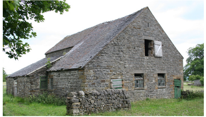
A combination barn characteristic of the Pennines with doors in the gable leading to feeding passages for cattle stalls which extended into projecting outshots (lean-tos). Photo © Jen Deadman
